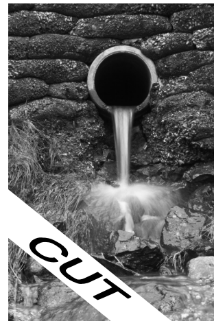
No water quality monitoring in many locations
